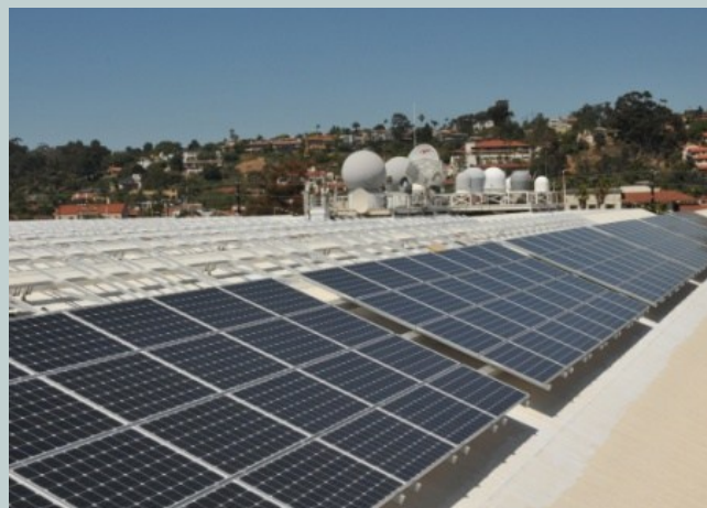
Solar panels installed on the roof of Space and Naval Warfare Systems Command Headquarters Old Town Complex in San Diego, California. (Photo by Rick Naystatt/Released)
