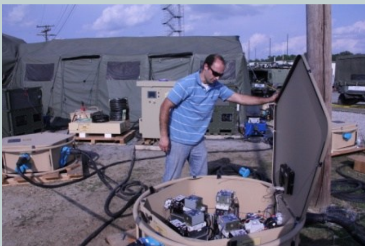
CERDEC demonstrated a proof of concept for a smart grid that could support tactical operations this summer at its integrated capabilities test-bed at Fort Dix, N.J. (Photo by Spc. Robert Porter/Released)
