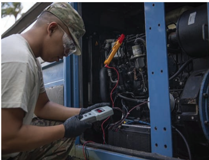
Figure 6-1. Staff Sgt. Gabriel Carias, 624th Civil Engineer Squadron, Conducts a Routine Maintenance Check on the Battery of an Electrical Generator at Bellows Air Force Station, HI, January 2020 (Source: Kurka [244]).
