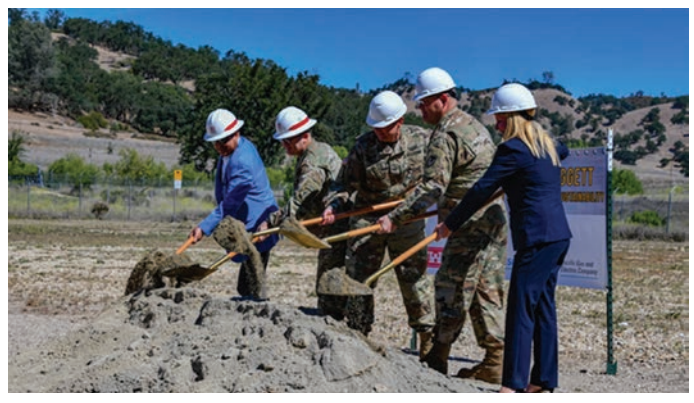
Figure 1-3. Leaders From Fort Hunter Liggett and Its Partners Ceremonially Break Ground on the Base’s Microgrid Project in May 2021 (Source: Croft [57]).
