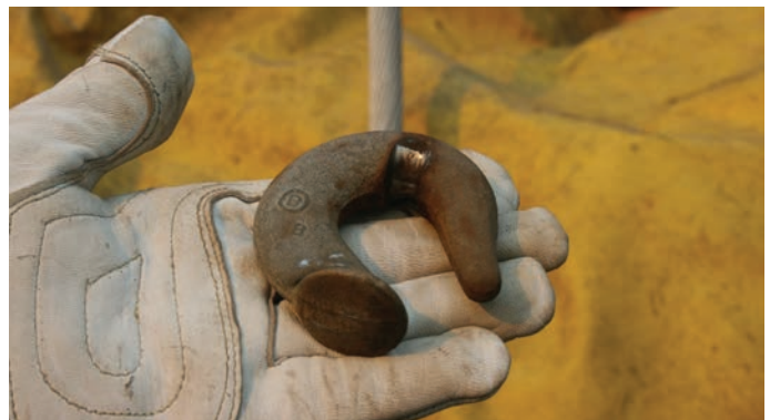
Figure 3-2. A C-Hook From Pacific Gas and Electric Company Tower 27/222 Shows Metal Channeling Due to Decades of Wear (Source: Long [137]).
