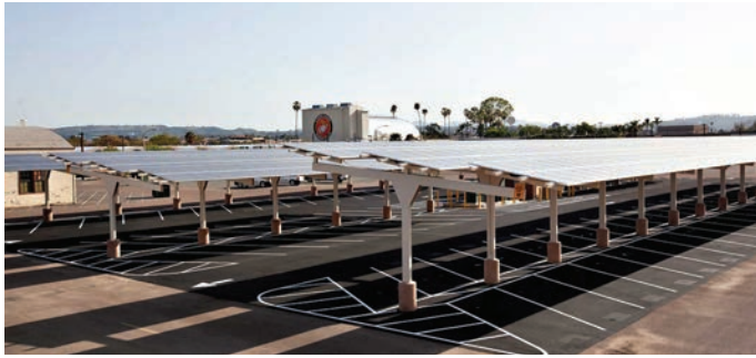
Figure 1-1. A 250-kW Section of Solar PV Modules Serves Double Duty at MCAS Miramar, Contributing to the Microgrid’s 1.3 MW of Solar PV Capacity and Providing Sun Protection for Parked Cars (Source: NREL [13]).
