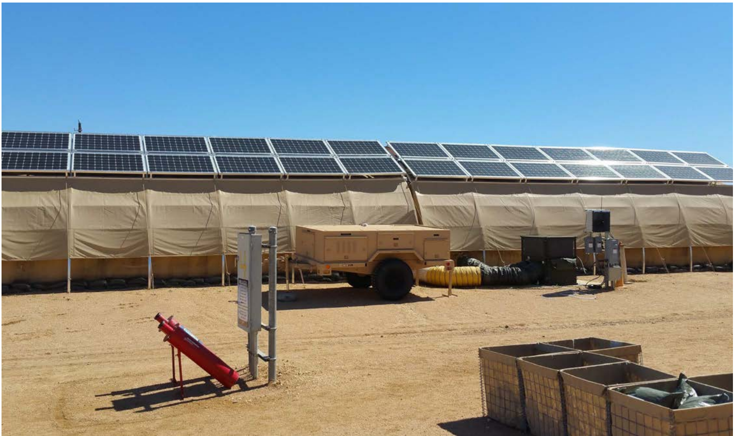
Figure 4. Monocrystalline Silicon Solar Panels Placed on Top of Each Tent for Energy Production. A Trailer (Center) Holds the Hardware, Software, and Lithium Ion Batteries That Form the Smart Grid and Provide Energy Backup Should the Grid Fail (Source: Photo by Donna M. Lindner, U.S. Air Force Research Laboratory).
